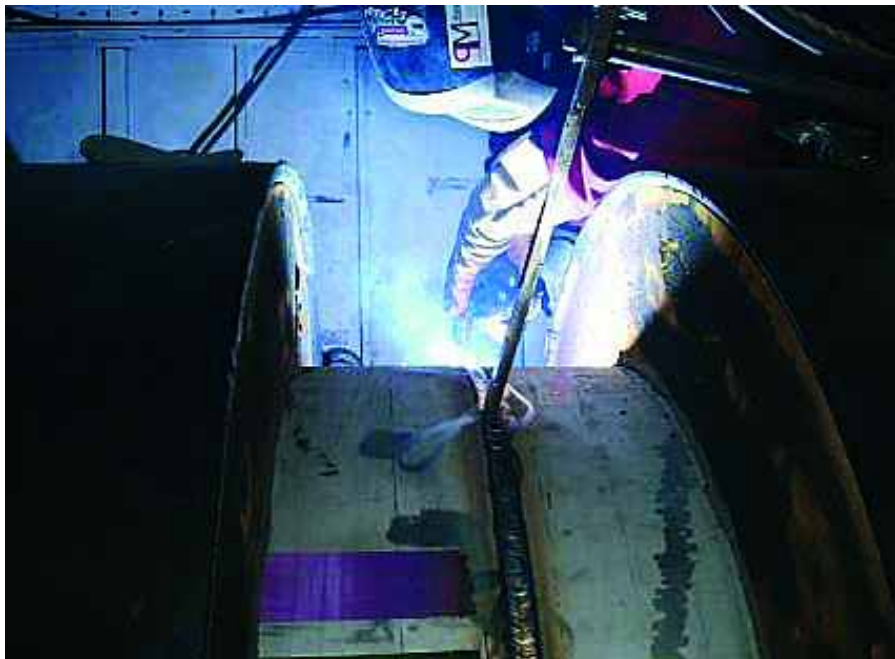
Figure 11: Gas shielded flux cored arc welding, controlled ferrite 308L, being used for the first time during construction of the Grain-LNG importation facility on the Isle of Grain, UK.
